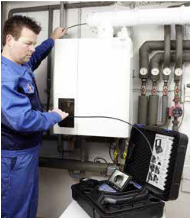
The service camera is an essential partner in a wide range of applications including the analysis of flue gas installations.
