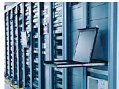
Control Room/ Data Center
