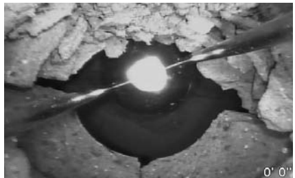
Figure 13 – Typical Crossbore Into Sewer Line
