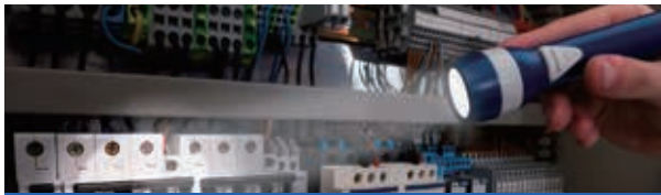
Erroneous circuit-breaker activation
