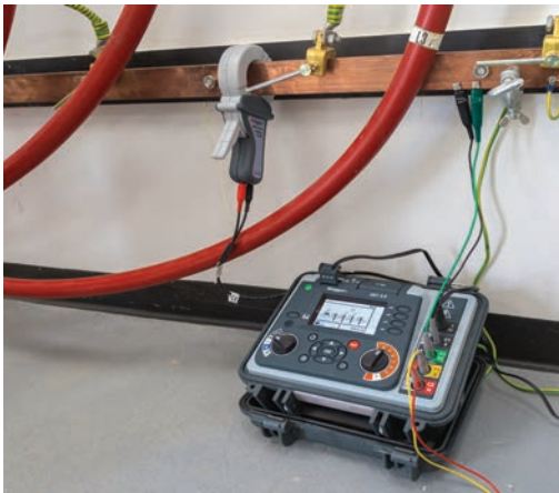
Using ART method with Megger DET2/3 Series to test commercial earth (ground) without disconnecting the system
