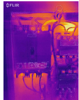
Identify electrical faults
