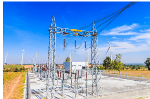
Substation partial discharge
