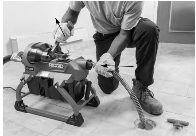
Figure 14B – Clutch Released, Cable Not Rotating, Feeding Cable Into Machine
