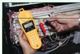
Telephone line testing
