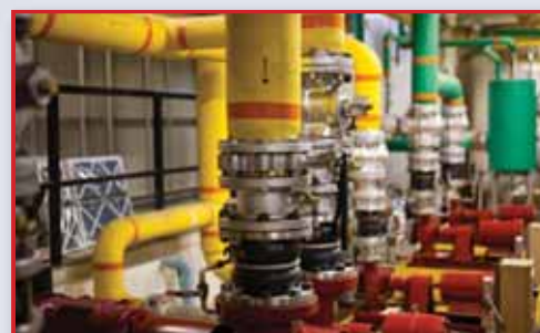
Boiler Room Pump Maintenance
