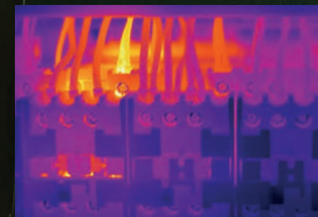
MAINTAIN SYSTEMS Identify excessively high temperatures in circuit breakers and electrical components before breakdowns occur.
