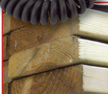
Check wood for dampness or rot
