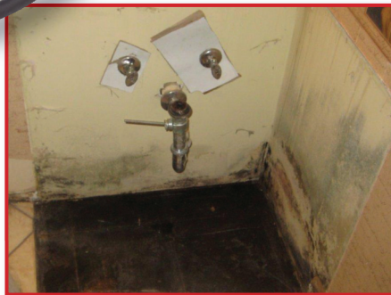
Locate moisture/water damage
