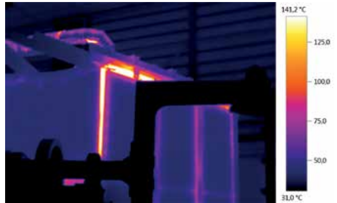
Industrial kiln with faulty insulation.
